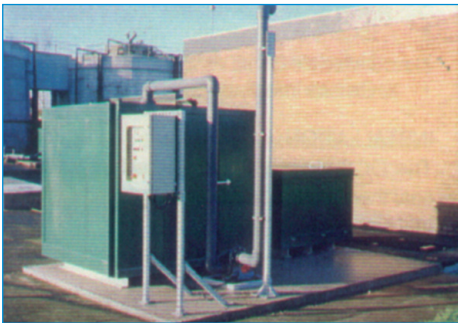
Peackmaker 3000 Module serving Imported Sludge and Return Liquors Well
