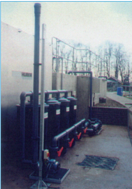
Peackmaker Modules in parallel serving small Works Inlet Area
